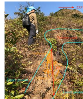
Figure 4d: Field photography of the tension crack
