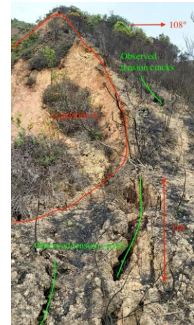
Figure 5d: Field Photograph of Landslide A
