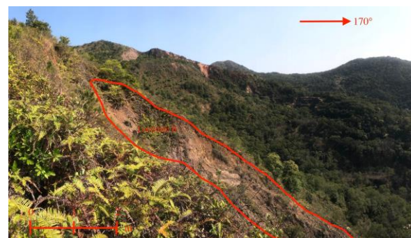
Figure 6d: Field Photograph of Landslide B
