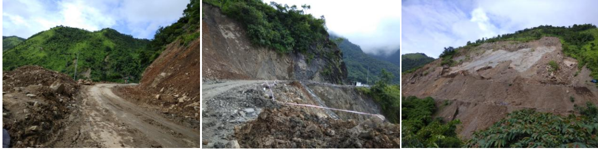
FIGURE 4: LANDSLIDE LOCATIONS COLLECTED DURING FIELD SURVEY
