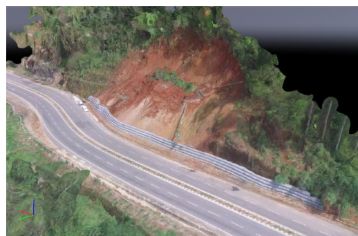
Figure 22: 3D View of Landslide Scar
