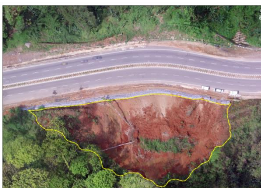
Figure 21: 2 D view of Landslide Scar
