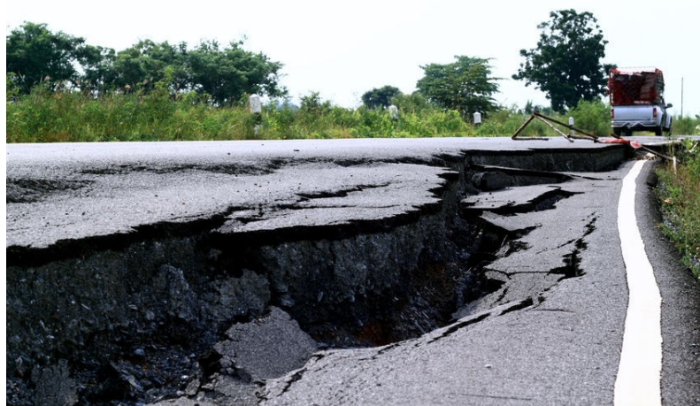
Figure 1. Road collapse example. (photo from 123rf.com )
