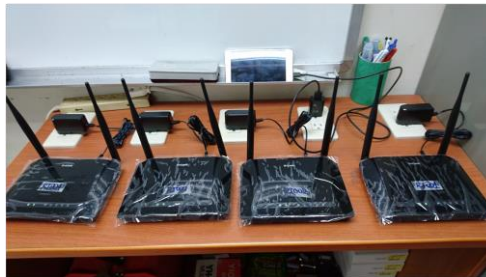
Figure 12 four same specification APs
