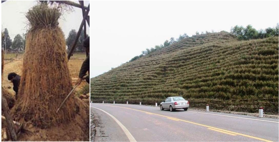
Figure no 3: roots of Vetiver grass and the planted grass to prevent the landslide and erosion.
