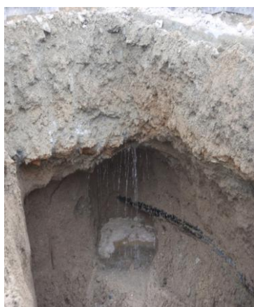
(a) Leak found at the area detected using GPR
