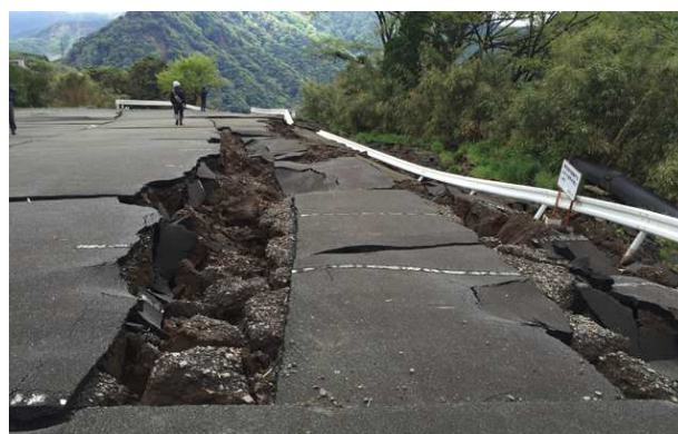
(b) Cracks in a parking place
